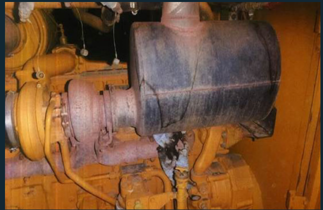
Engine fire caused by rag placed on hot surface. Image sourced from Resources Safety and Health Queensland.
