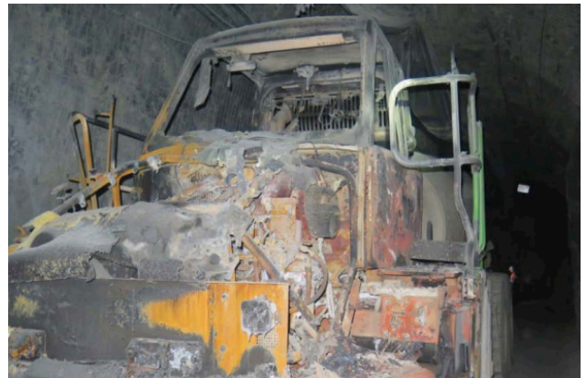
Underground fire fuelled by diesel and non-metallic materials. New South Wales Resources Regulator Fires on Mobile Plant, April to June 2019.
