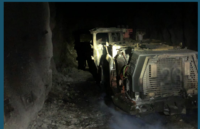
Broken wire to brake solenoid causes fire to loader being operated under tele-remote conditions. New South Wales Resources Regulator Fires on Mobile Plant, April to June 2020.
