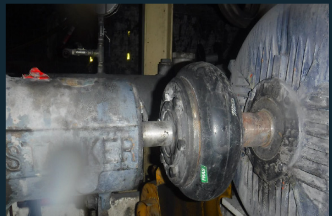
Underground pump fire. Image sourced from Resources Safety and Health Queensland .
